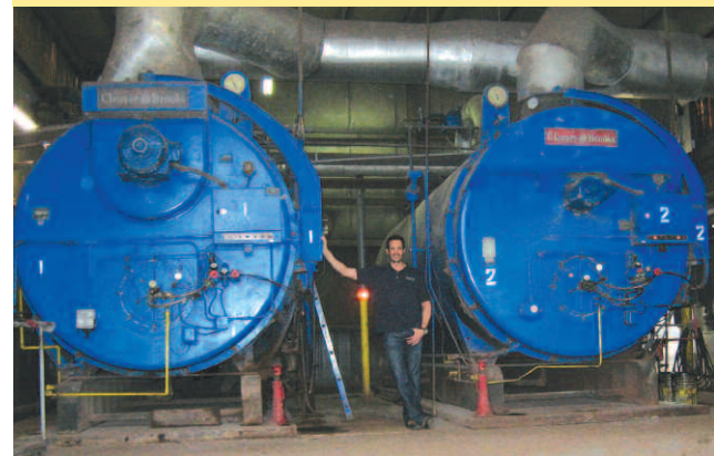
Matt standing by two 600 HP, low-pressure steam boilers at Olson's Greenhouses. The boilers are large enough to park several Hummers inside.
